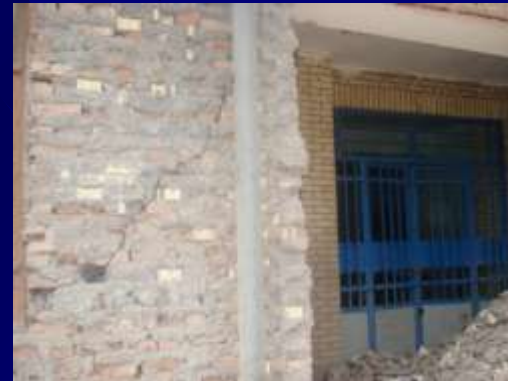
Diagonal cracks in masonry pier between two openings
