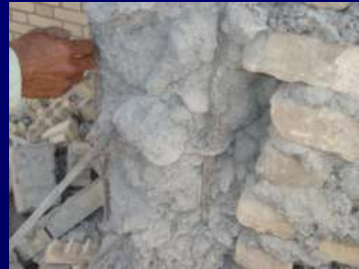
poor quality RC column with steel bars exposed
