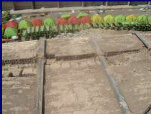
Anchor bolts for steel I-beams
