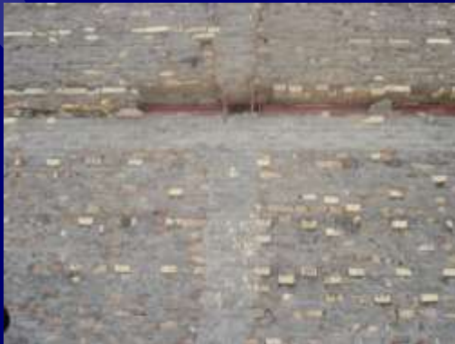
Poor quality masonry and columns bars exposed at floor level
