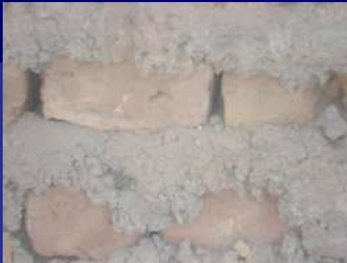
Poor quality masonry with too thick mortar joints
