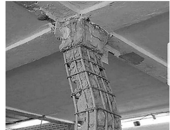
Instability (Due to deformations e.g., Buckling)
