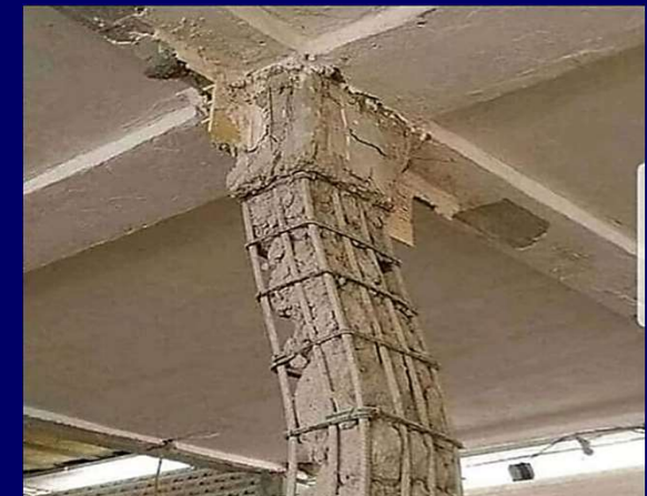
Instability (Due to deformations e.g., Buckling)
